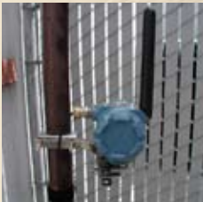
Mesh Wireless Link to the Control Room
