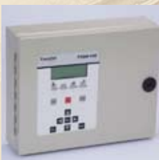
Familiar TraceTek Alarm Panel in Control Room
