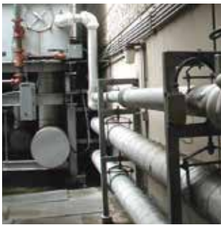
Pipe Freeze Protection
