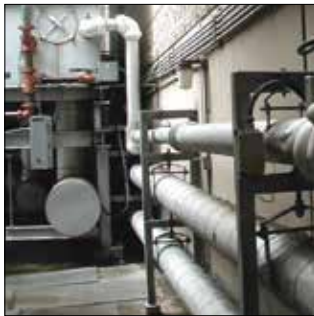
Pipe Freeze Protection
