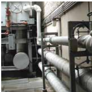
Pipe Freeze Protection
