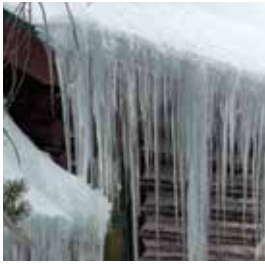
Unprotected roof and gutters
